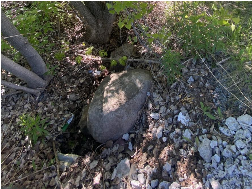
Photo 10. Photo taken of the outfall channel before it crosses under a grave side road running along the north side of the WTP building.
