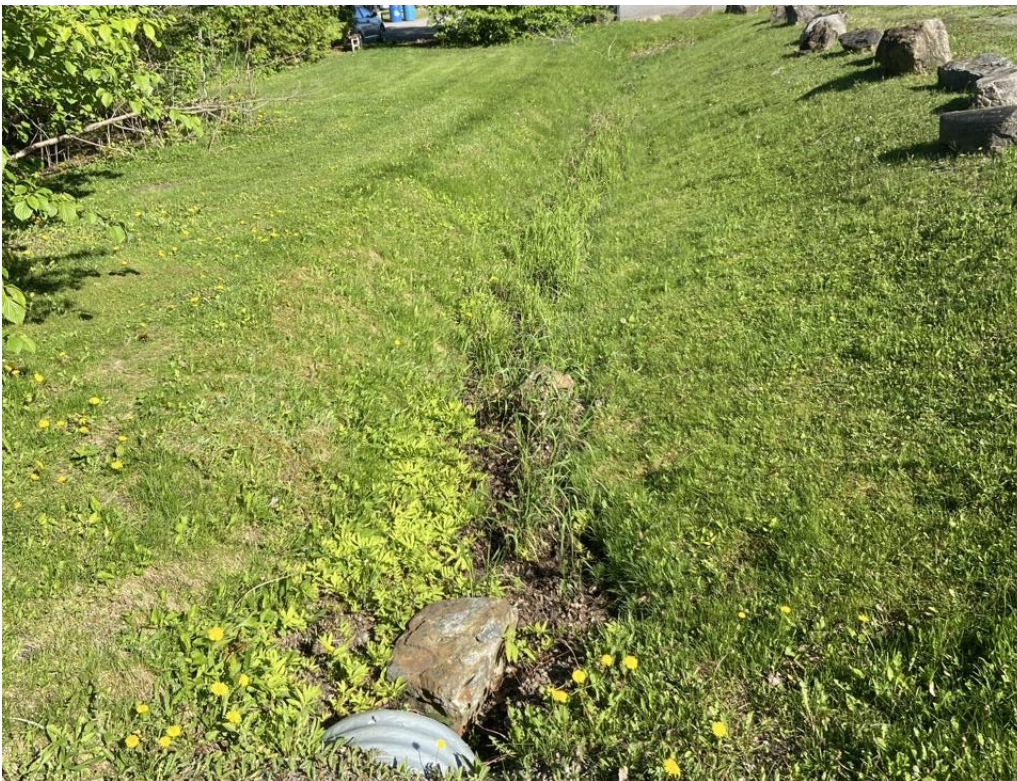
Photo 12. Photo taken facing north, showing the outfall channel after it crosses under the gravel side road.
