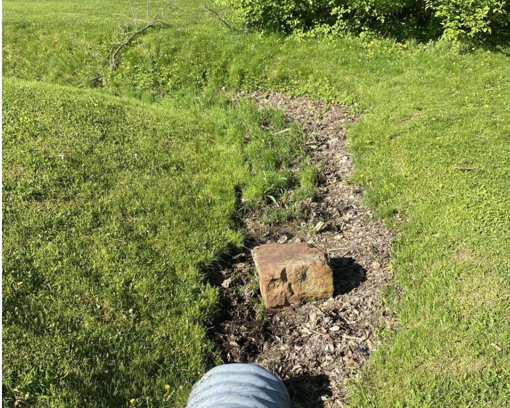
Photo 13. Photo taken facing west of the outfall channel before it crosses under a second gravel road that provides access to the back of the WTP.
