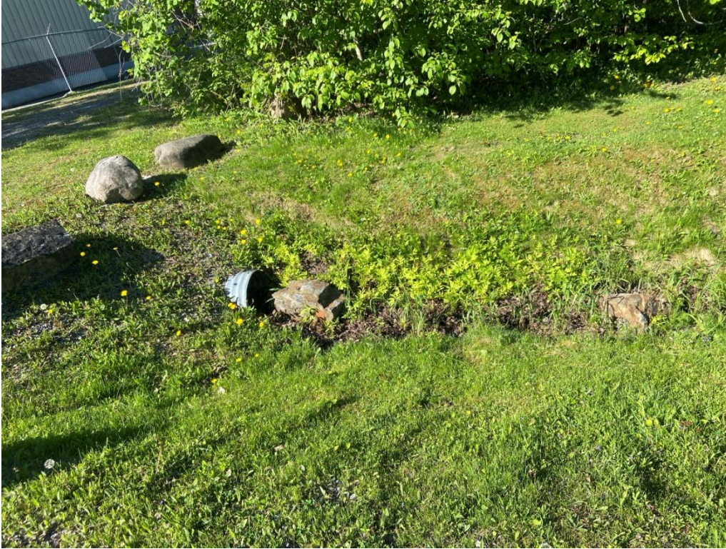
Photo 11. Photo taken facing west, showing the outfall channel after it crosses under the gravel side road.
