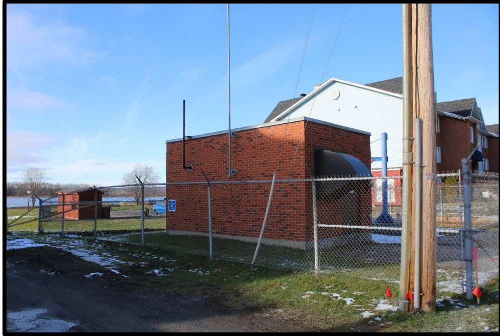
Figure 30. Sewage Pumping Station, Edwards St. Matrix Heritage, Nov 19, 2025.
