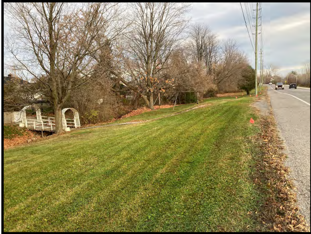
Figure 37: Buried utilities visibly marked along the road, steep slope down to ditch/creek. (MH1125-D137)
