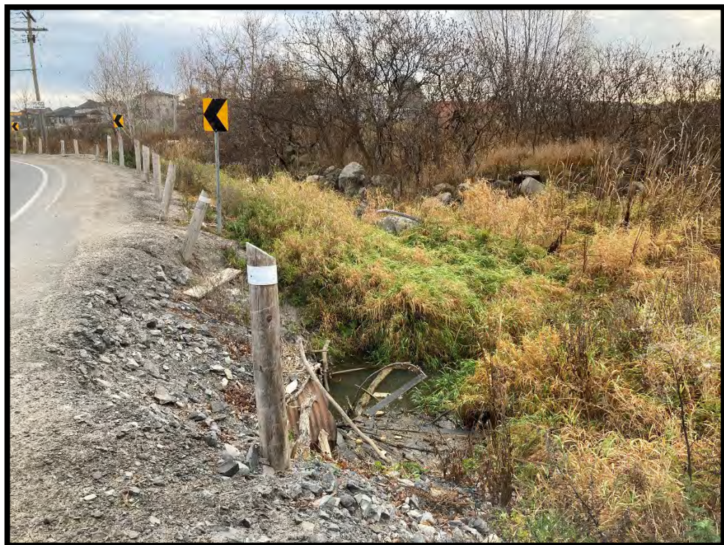
Figure 46: Disturbed soil, debris, fill, culvert and drain for creek into marshland in central portion. (MH1125-D120)
