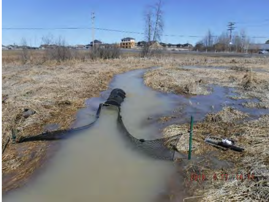
Photo 3 : Showing the extent of the overtopping of the banks on the downstream side St Jean Street (April 17, 2019)
