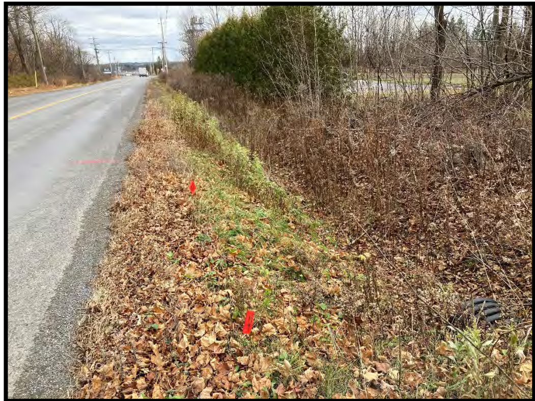
Figure 16: Ditch on the southern side, near dog park, showing buried Hydro lines. (MH1125-D240)
