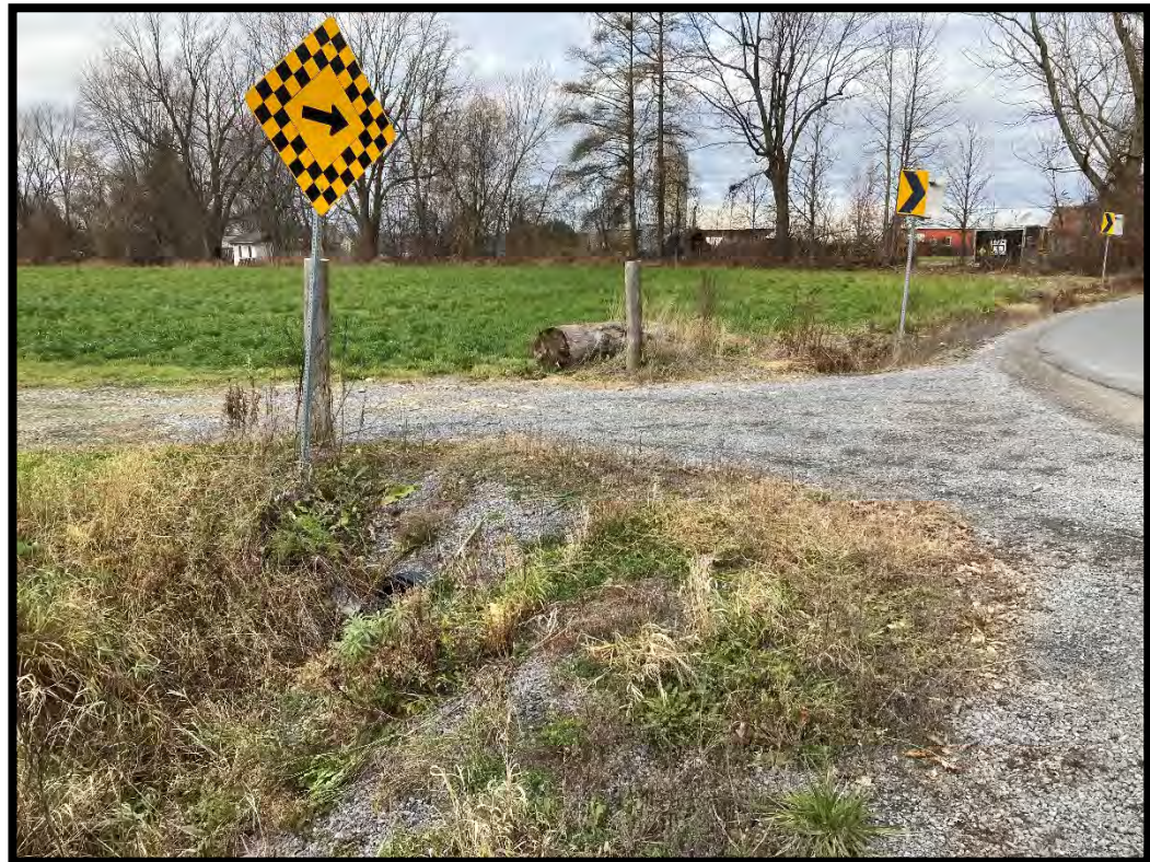
Figure 52: Western extent of the study area, gravel shoulder, culvert, wet conditions. (MH1125-D207)
