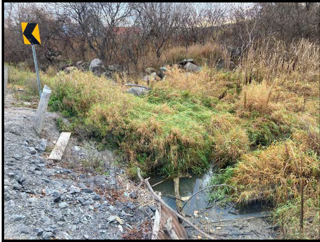
Figure 21: Debris and culvert with creek flowing into the marsh. (MH1125-D118)
