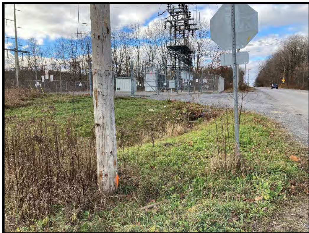
Figure 2: Hydro station with ditch and drain. (MH1125-D141)
