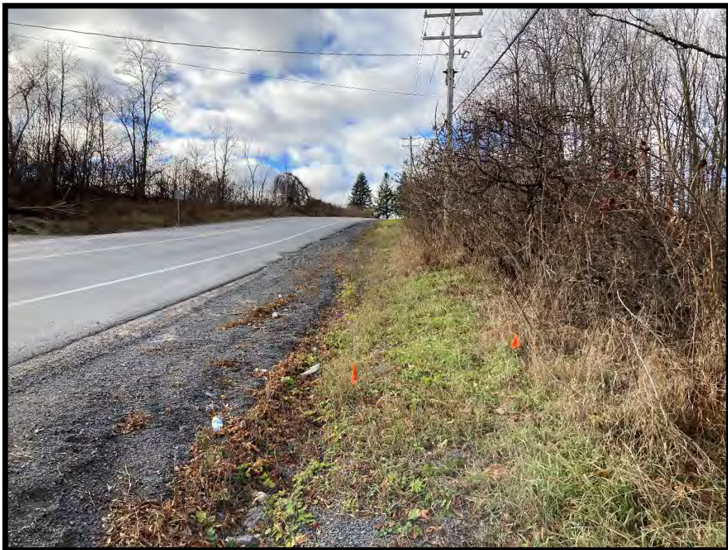
Figure 18: Berm and slope up to western side of the study area with buried utilities. (M1125-D155)
