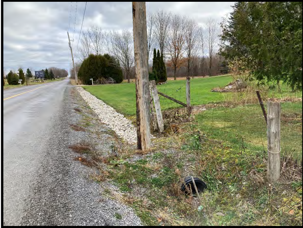
Figure 53: Western portion of study area, south side of the road, ditch, gravel shoulder, fill. (MH1125-D211)
