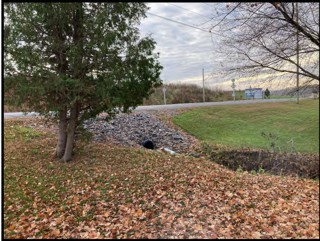
Figure 45: Culvert and drain with large stone gravel into creek on western side. (MH1125-D057)
